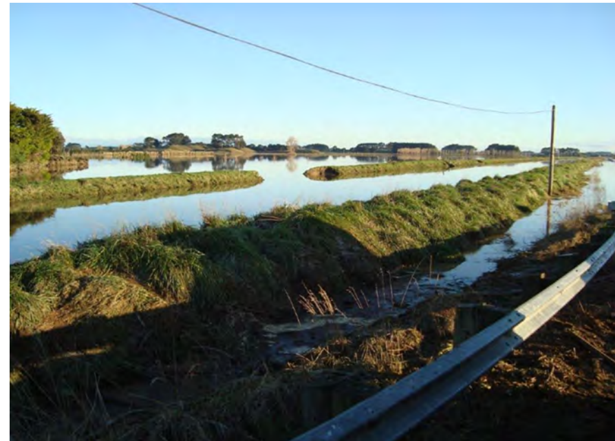
Figure 19: Example of asset failure. Stopbank breach in Sluggish Main Drain in the Te Kawau Drainage Scheme during the 2015 flood event.
