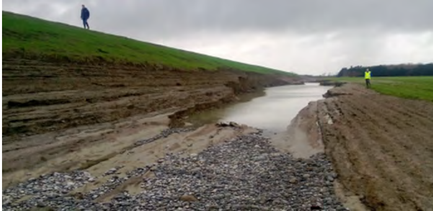
Figure 8: Inspection of a stopbank damaged during a storm event. Climate change is likely to increase the amount of asset inspection and repair work required.
