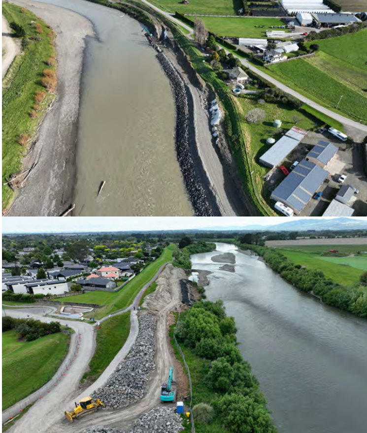
Figure 12: Photos in two flood protection upgrades completed as part of the Climate Resilience work programme. Above: rock armouring at Te Matai Road, Manawatū River. Below: Albert Street, Palmerston North.
