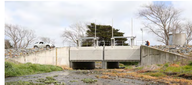
Figure 25: Asset condition inspection at the Makino flood gates upstream of Feilding. This asset is an example of high criticality asset.
