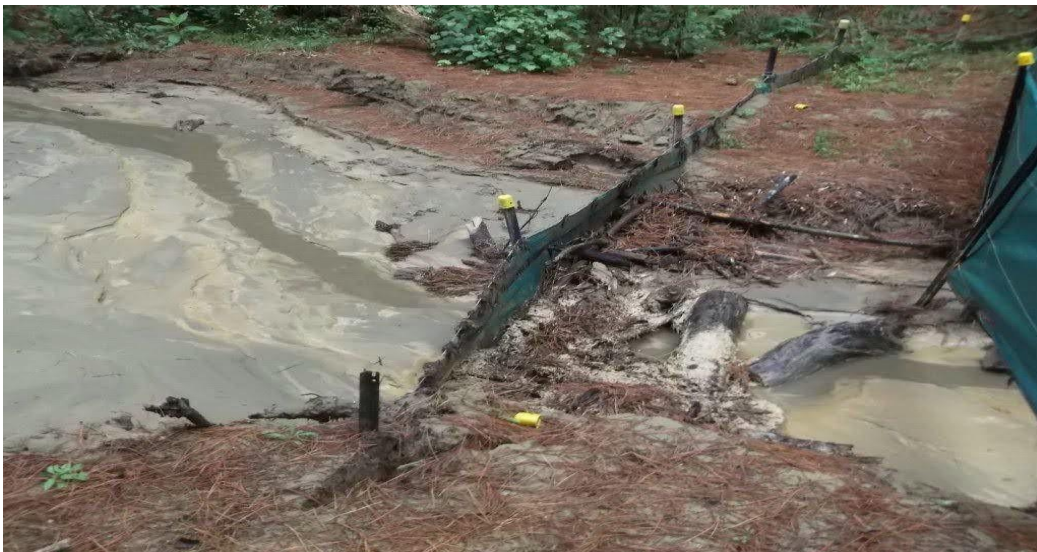
A reasonably effective debris dam in unconsolidated sands Whanganui catchment. Note dam goes right up the bank so water cannot cut around the side.
