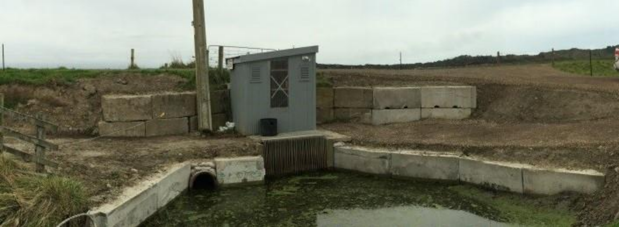
Photo – Duck Creek pumpstation
